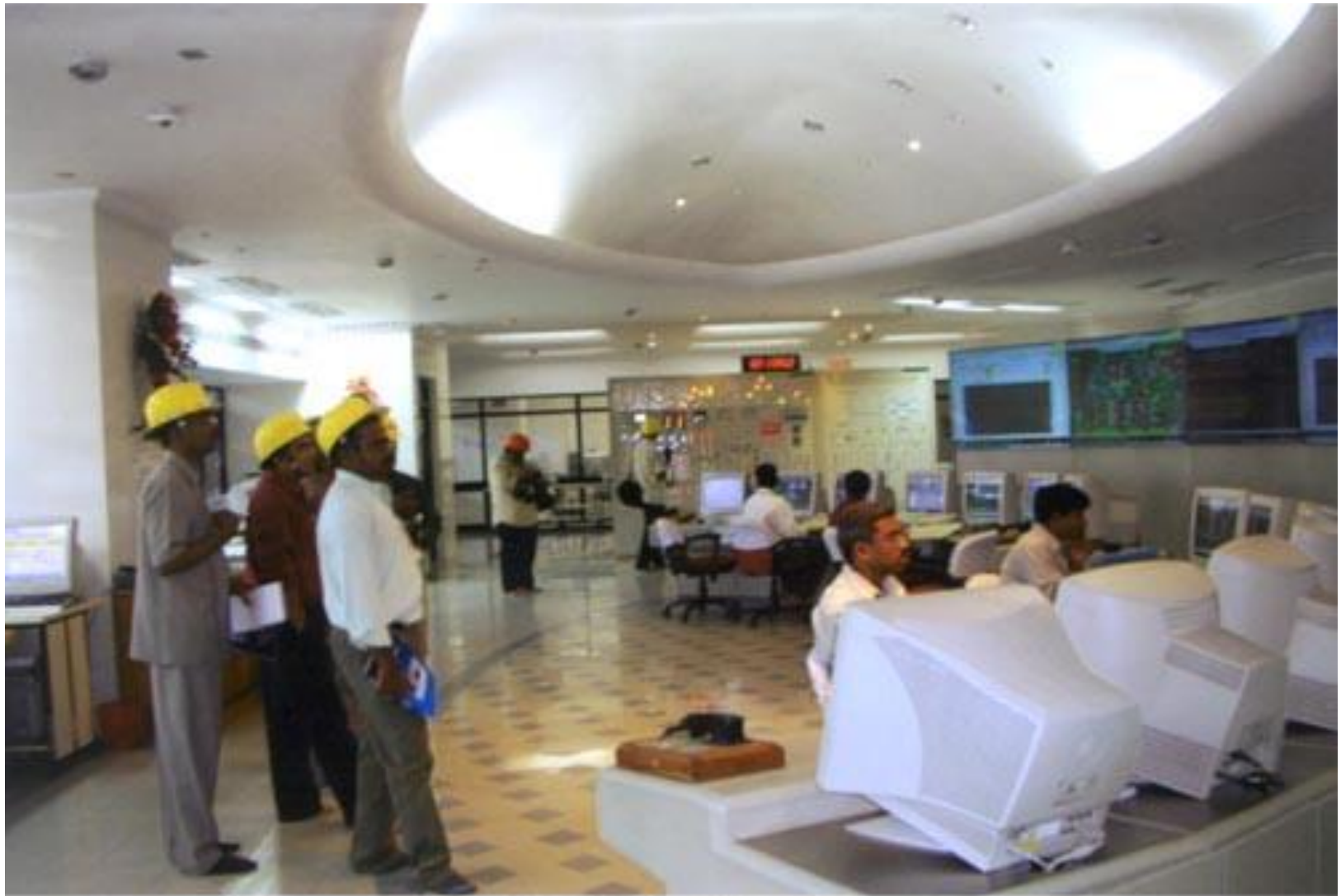
The state-of-the-art control room in the Simhadri Thermal Power Project
